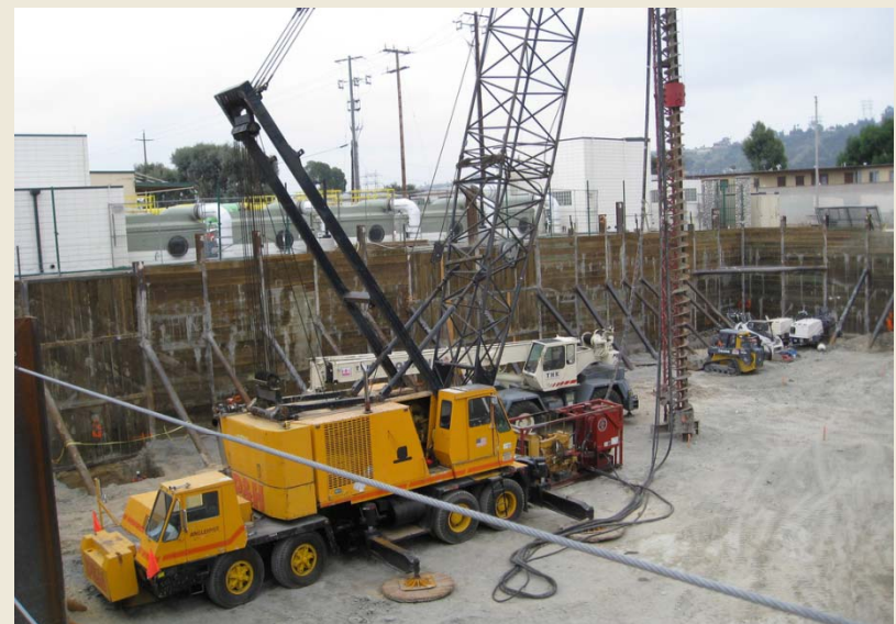
Looking east from the La Brea Aerial Station (t) and construction of La Cienega Parking Structure (b)
