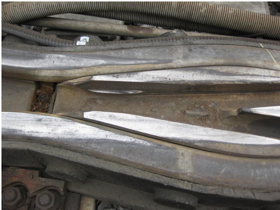
Figure 7: Observed Wing Rail Wear
